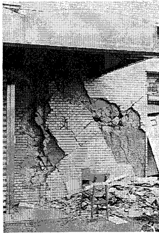
Photo 4 Damage to shearwalls in an older RC building
