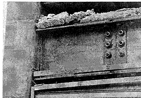
Photo 13 Failure of a beam-to-column connection
